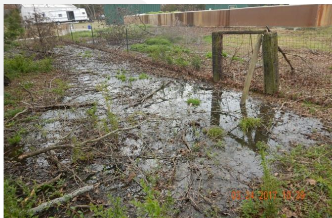
Before – Sewage overflow
