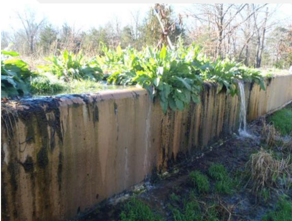
Before – Vegetation and sludge in sand filter
