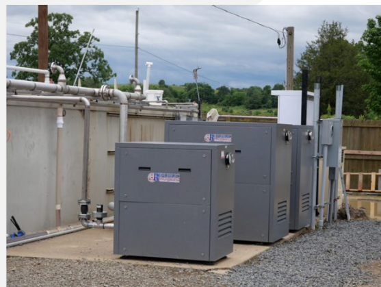
After – New treatment equipment
