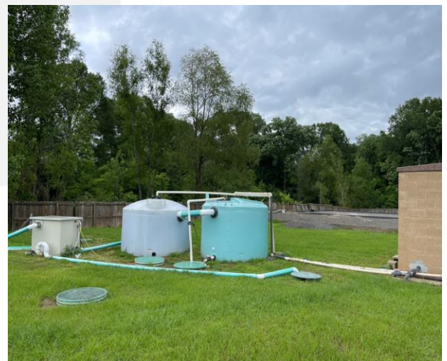
After – MBBR treatment system
