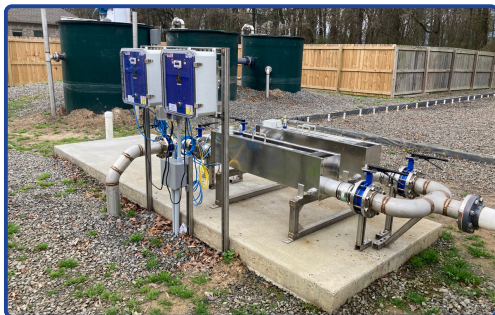
UV Disinfection System
